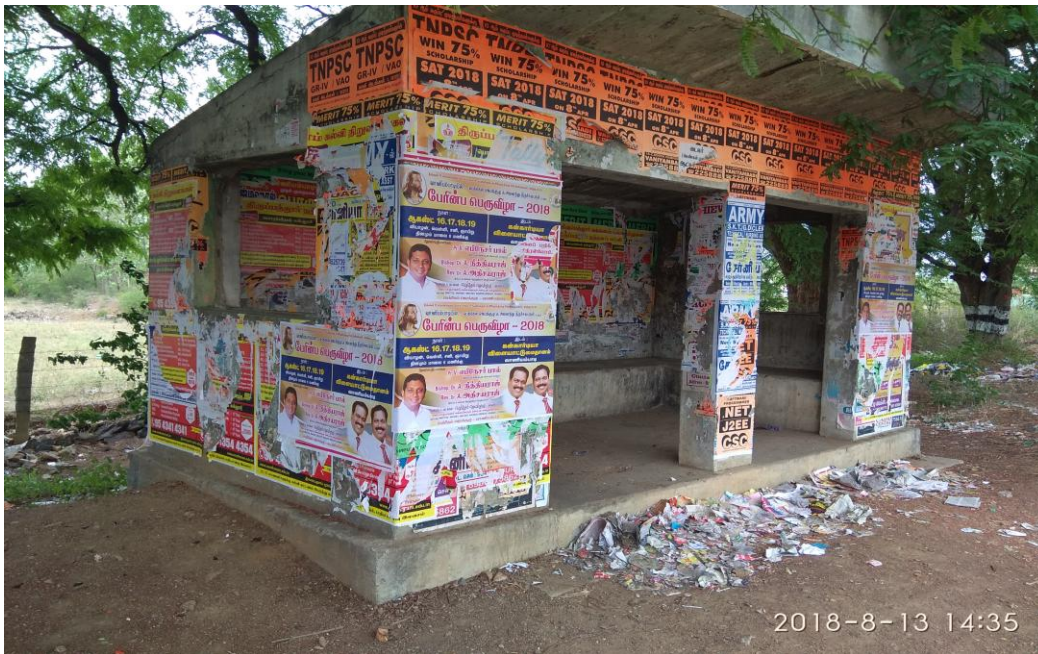
Bus stop before cleaning
